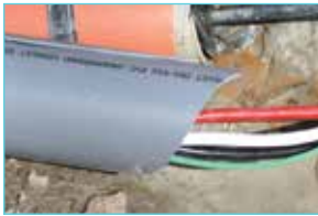
BROKEN SECTION OF DUCT
