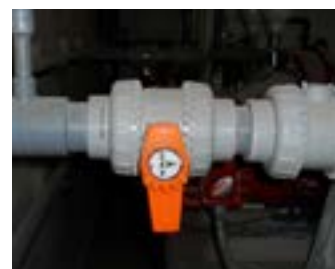
IPEX manual VXE, VX and electric actuated VKD Series Ball Valves were used throughout the facility to control flow as needed.
