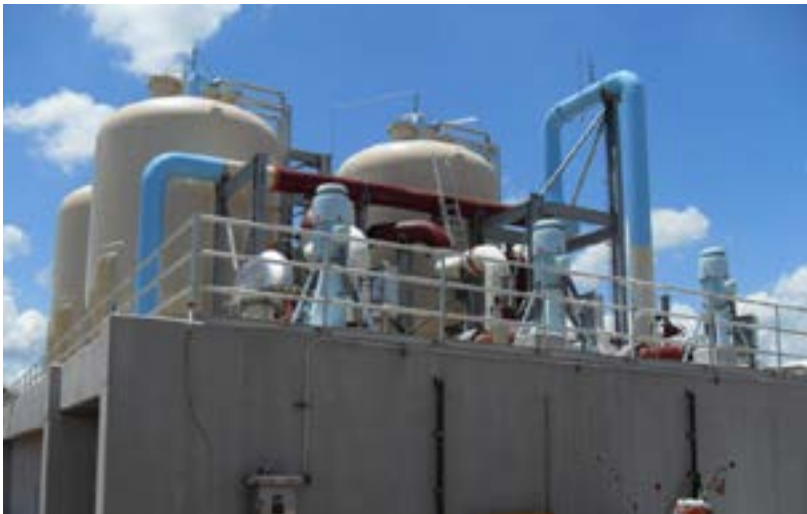
The City of Sugar Land Surface Water Treatment Plant delivers 9 MGD of potable water to residents.
