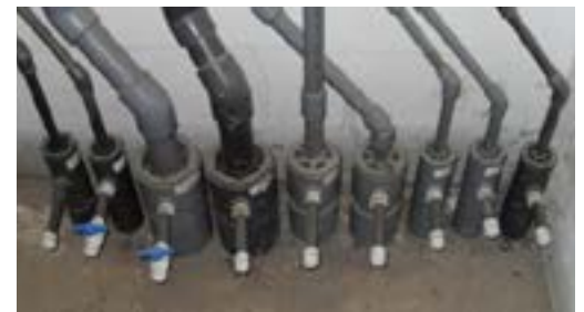
The IPEX Guardian™ Vinyl double-containment system was required for underground runs, which transitioned to IPEX single wall PVC and Xirtec® CPVC inside the facility.
