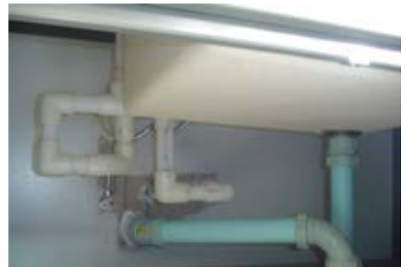
IPEX Enpure™ was used for high purity processing of water and reverse osmosis distribution system
