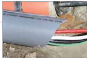
BROKEN SECTION OF DUCT
